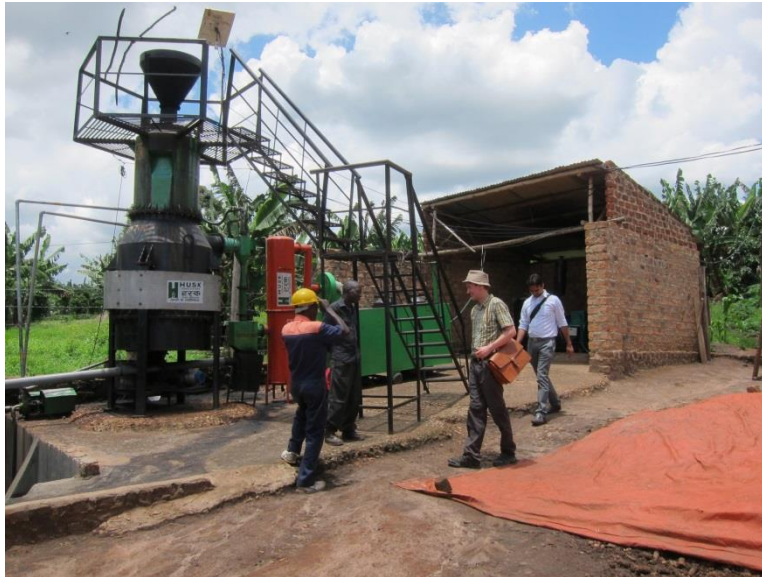
A gasifier in rural Uganda providing basic electricity services.
